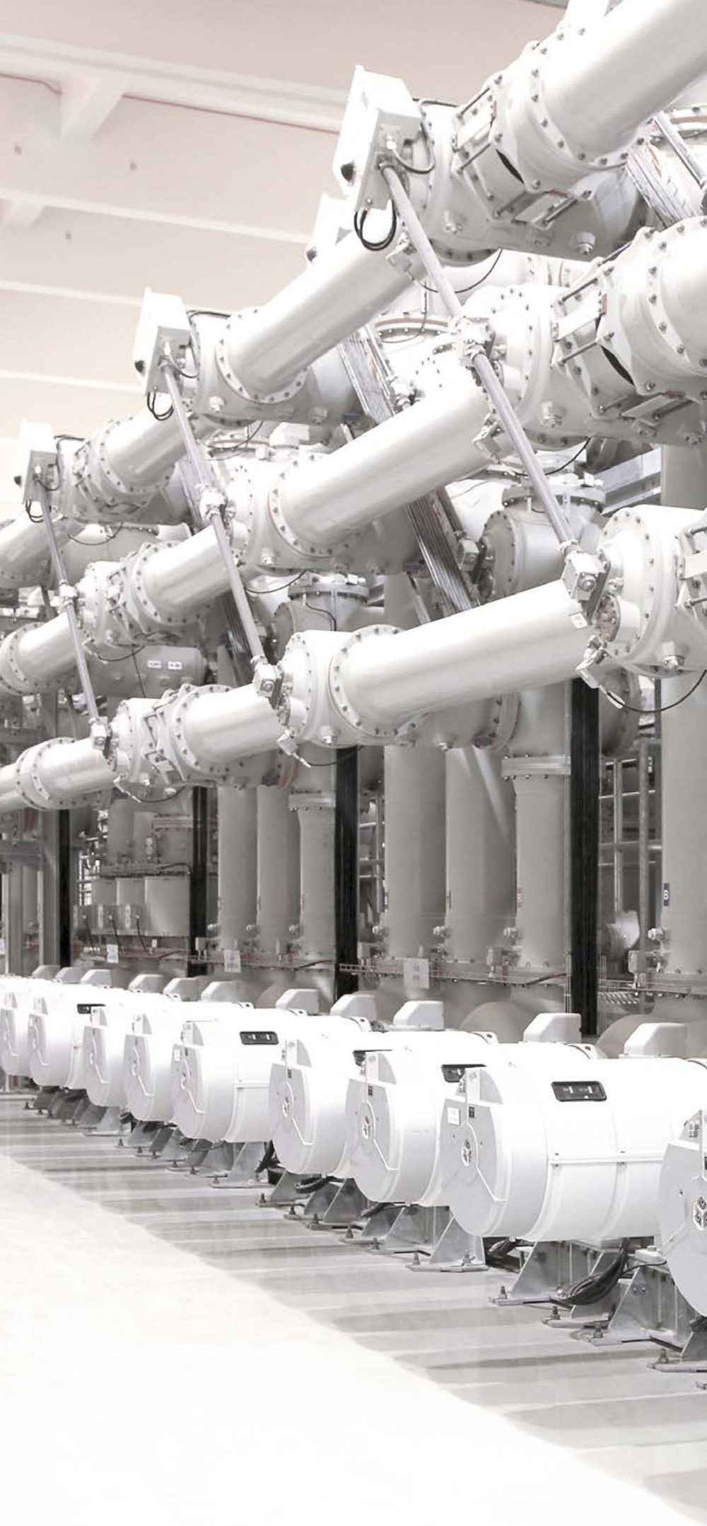
Gas-insulated switchgear (GIS) 400 kV, Qatar 2009 © Hitachi Energy
